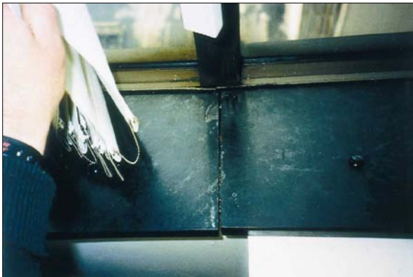
Asbestos Window Cill
