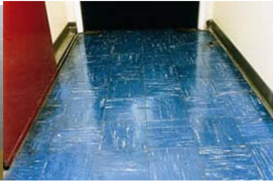
Asbestos Vinyl Floor Tiles
