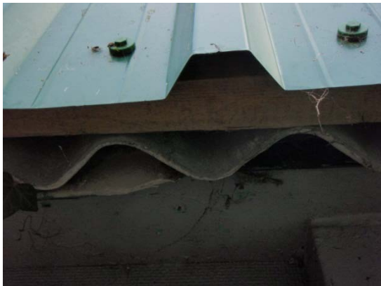
Asbestos Cement behind metal profile
