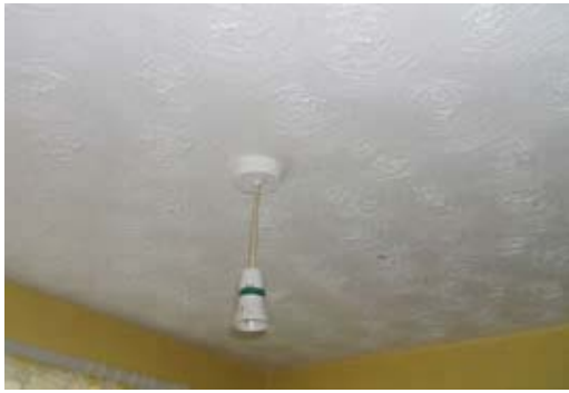
Asbestos Textured Coating (Artex) Ceiling
