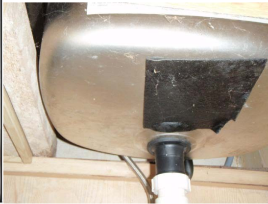
Asbestos Bitumastic Dampening Pad on Steel Sink
